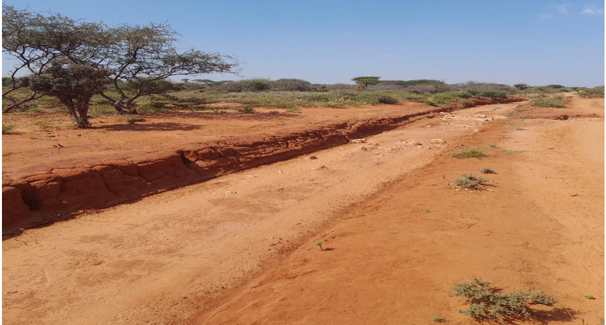
Figure 7. Channelization at some-section of the road
